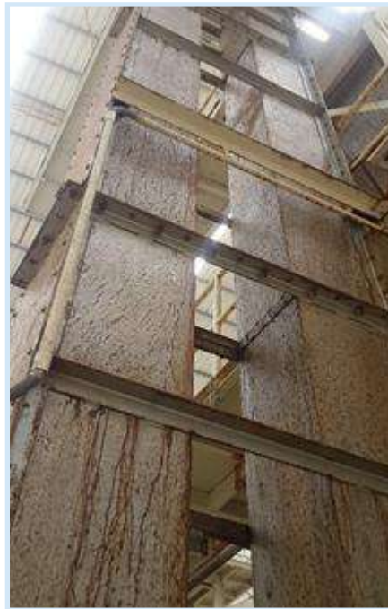
Closed system - cannot be cleaned
