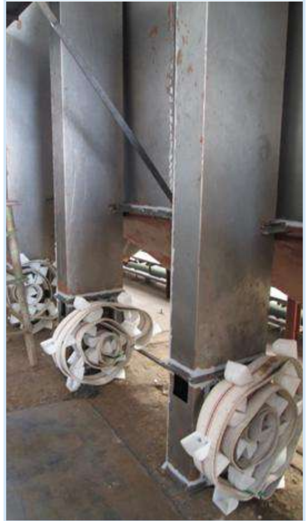
A battery of friction driven bucket elevators used in elevating tea leaves
